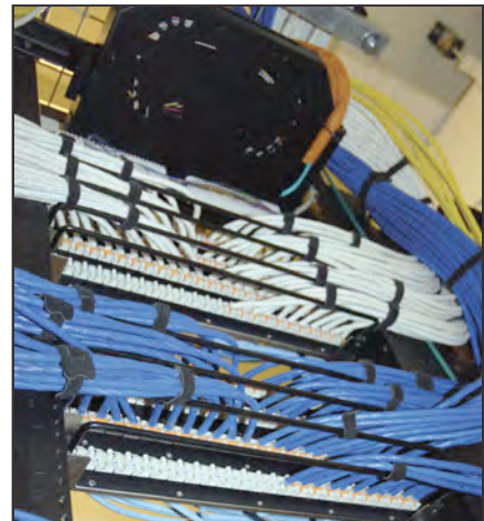
Belden's FiberExpress fiber backbone (Orange cable) runs from the Computer Room to each floor's telecommunications room. The 10GX copper-based cables (Blue, White and Yellow) run horizontally to deliver high-bandwidth 10 Gigabit to desktops on all floors. All fiber links have redundant pathways built in to ensure maximum reliability and network uptime.
