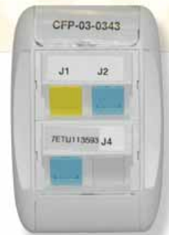
Each workstation in the Operations Support Building II is equipped with a MediaFlex face plate and three Belden IBDN System 10GX cables — two for data, one for voice. To date, 4,000 drops have been tested and all performed beyond 625 MHz without a single failure.
