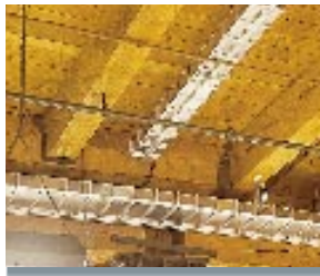
Open ceiling installation routed through cable trays.
