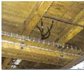
A close-up of a cable tray in an open ceiling installation.
