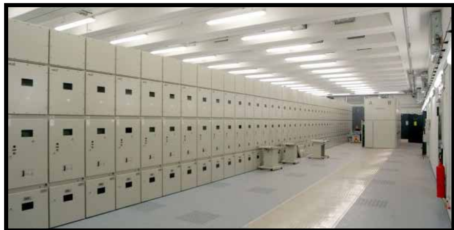
View into the depths: The 10 kV control cabinet room of the new substation is located approximately 17 meters below the surface.
