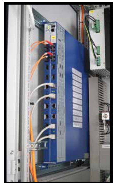
The substation used a MACH1000 Industrial Ethernet Switch in a vertical installation in the control cabinet.
